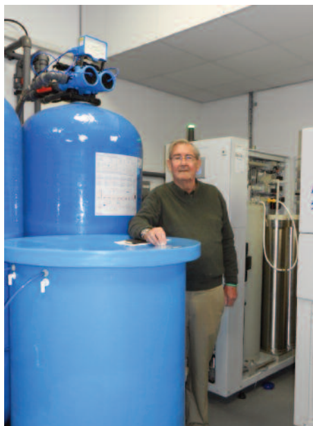
Peter Constable visiting the water treatment plant of the new unit on Open Day last December
